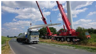
Assembly of rotor blades coated with riblet paint. © Mertcan Bayar, E.ON Climate & Renewables, Sweden
